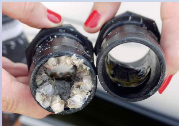
marine raw water line
